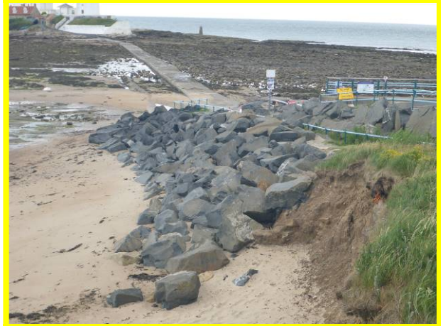
Erosion adjacent to rock revetment by St Mary's Island causeway (/4401C24 & 25)
