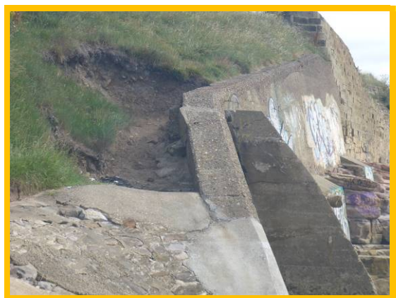
Erosion above wall (/4801C06)
