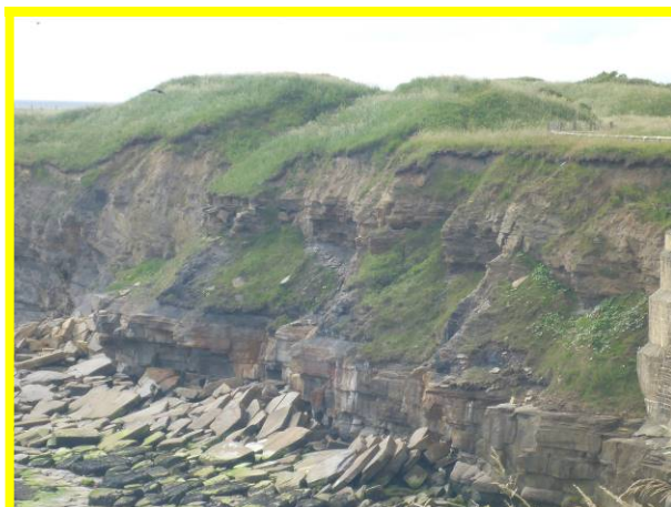
Rock falls in hard material along lower cliffs (/4401C24)
