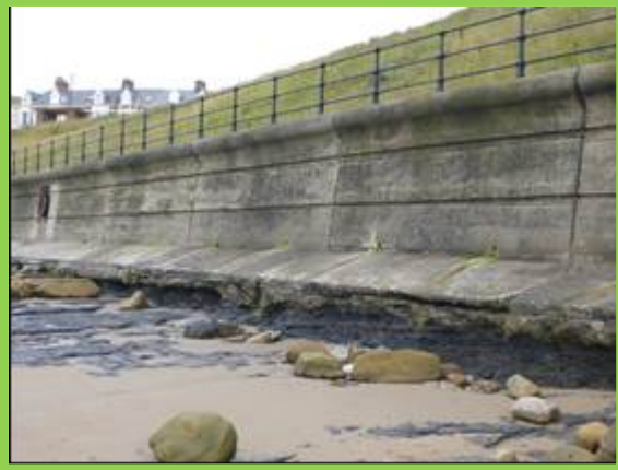
Undercutting and exposure of coal at toe of wall from 2018 inspections (/4701C18)
