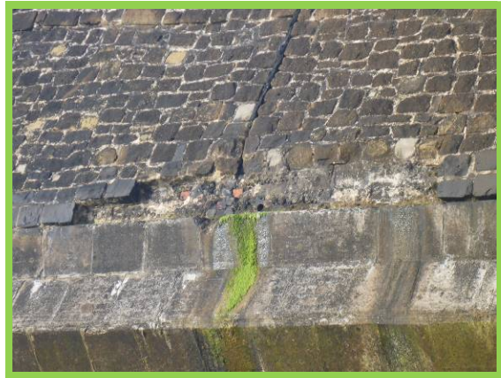
Missing brickwork (/4601C05)
