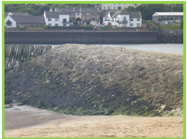
Erosion above wall (/4801C10)
