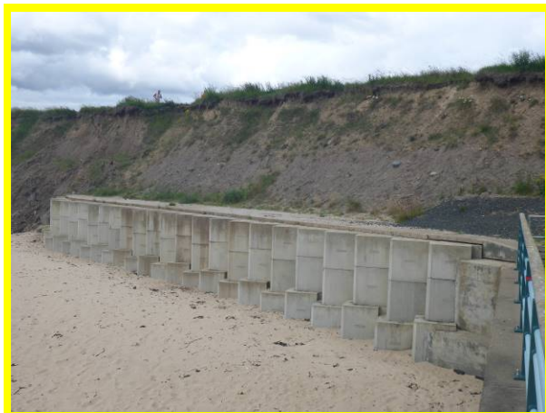
New T-Block units (constructed in 2014) prevent outflanking at the southern end of Trinity Road seawall (/4501C05)
