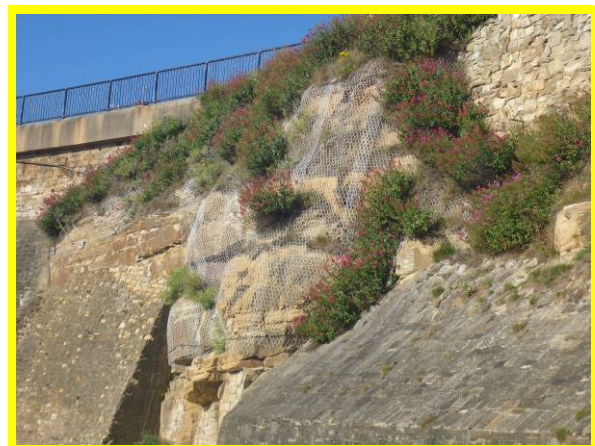
Rock bolts and netting on slopes to rear of promenade (/4701C01)
