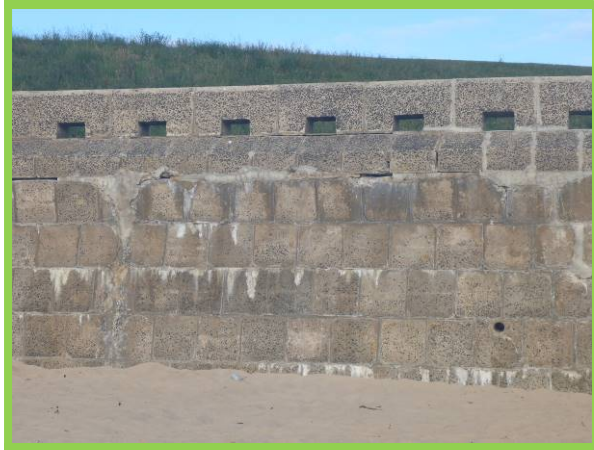
Previous repairs and local open joints which would benefit from maintenance (/4501C07)
