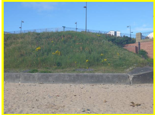
Concrete wall, blockwork revetment and slopes south of beach access ramp (/4601C01)
