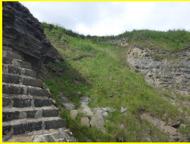
Slippage from 2009 in soft material adjacent to Hartley Cove access steps (/4401C22)
