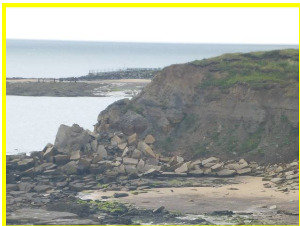
Slippages in soft material along upper cliffs and rock fall at base (/4401C22)
