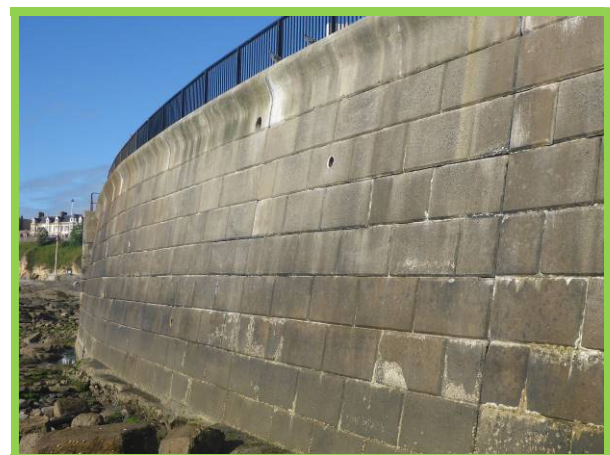
Middle section of sea wall in generally good condition but with face abrasion (/4701C05)
