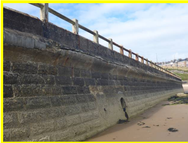
Wall abrasion at the Outdoor Pool (/4701C24)
