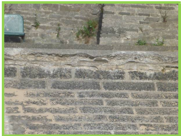
Abrasion damage to the revetment crest (/4701C19)
