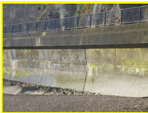
Brown's Bay southern sea wall in generally fair condition (/4701C01)
