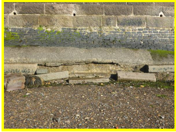
Some defects at the toe apron (/4701C06)
