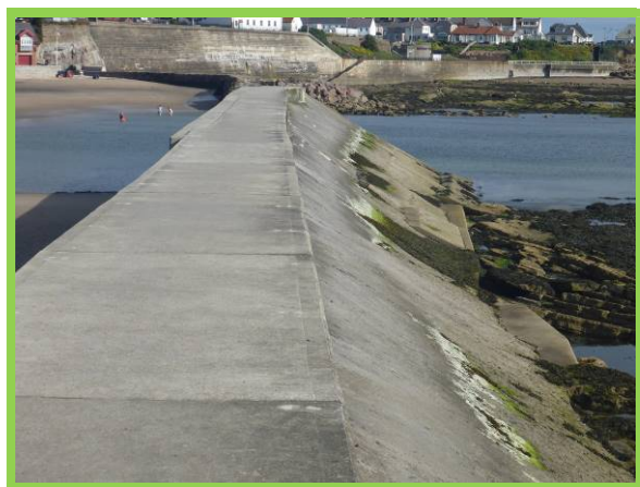
Cullercoates South Pier – sloping seaward face (/4701C15)
