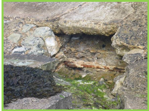
Damaged apron (/4701C27)
