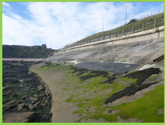
Sea wall in fair condition with damage and abrasion of the apron (/4701C27)
