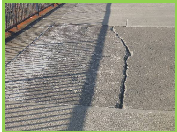
Surface cracks in promenade deck at northern end (/4601C10)
